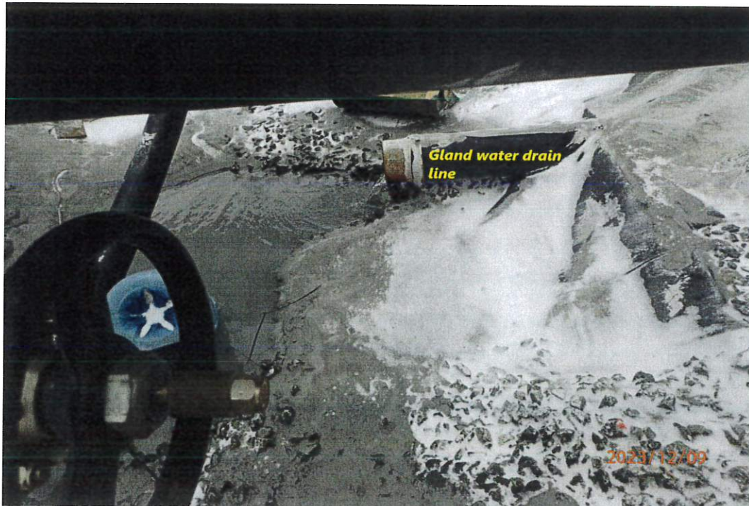
Figure 1: Gland water drain line and Booster Station.
