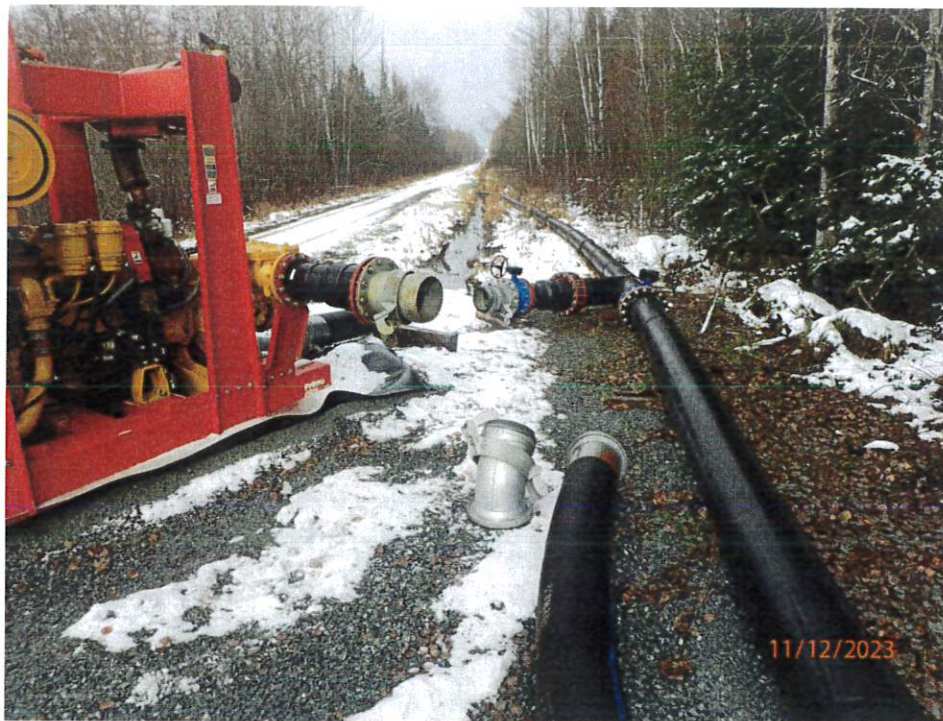
Figure 1: EDL2 Booster Pump and spilled effluent water in the ditch beside old Loslo Road.
