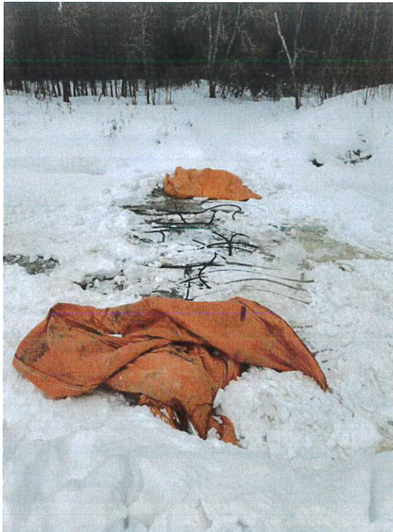
Photo 1: Chewed glycol line trapped in ice morning of February 27, 2023.
