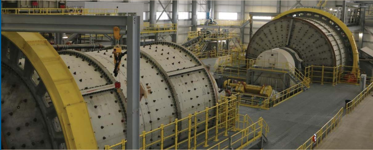
Semi Autogenous Grinding Mill (SAG Mill)
