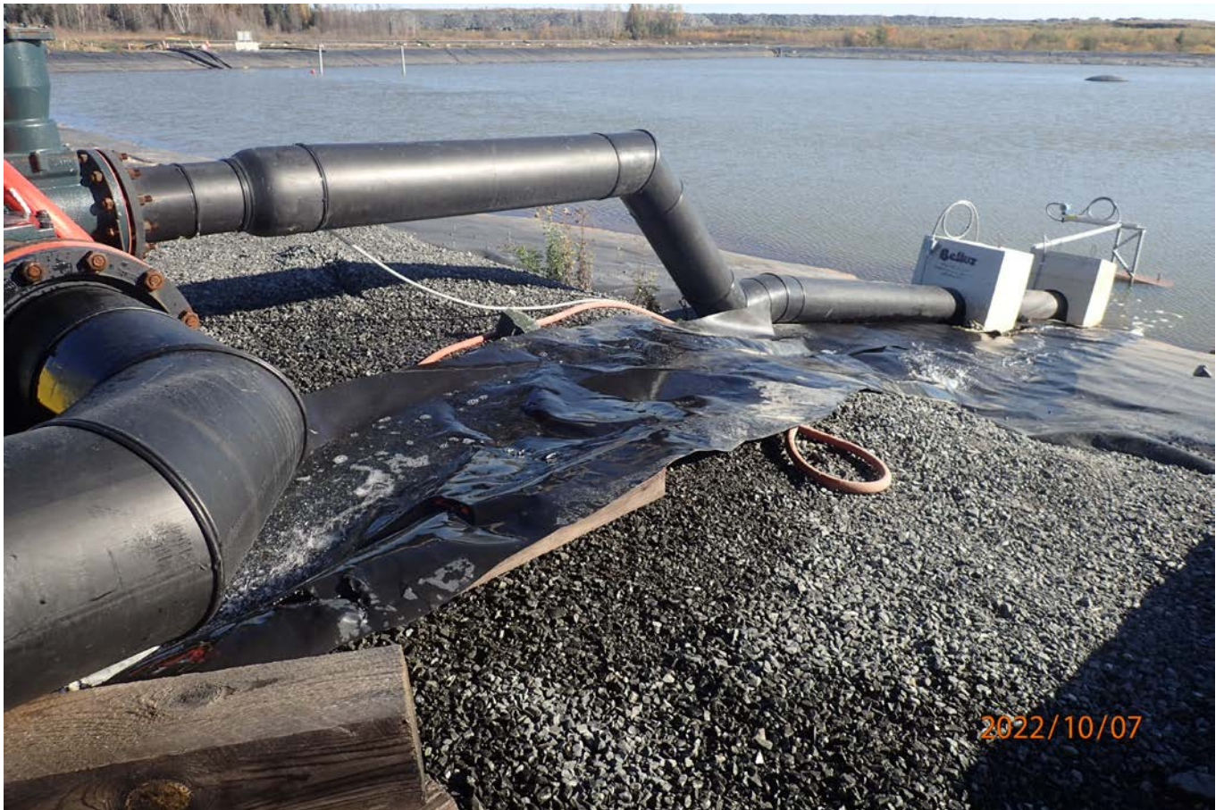
Photo 2; Scrap liner used to catch spill.
