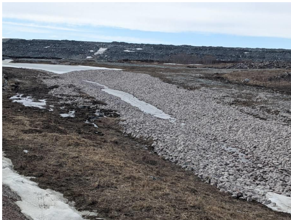
Figure 4 TMA seepage pond spillway activated.
