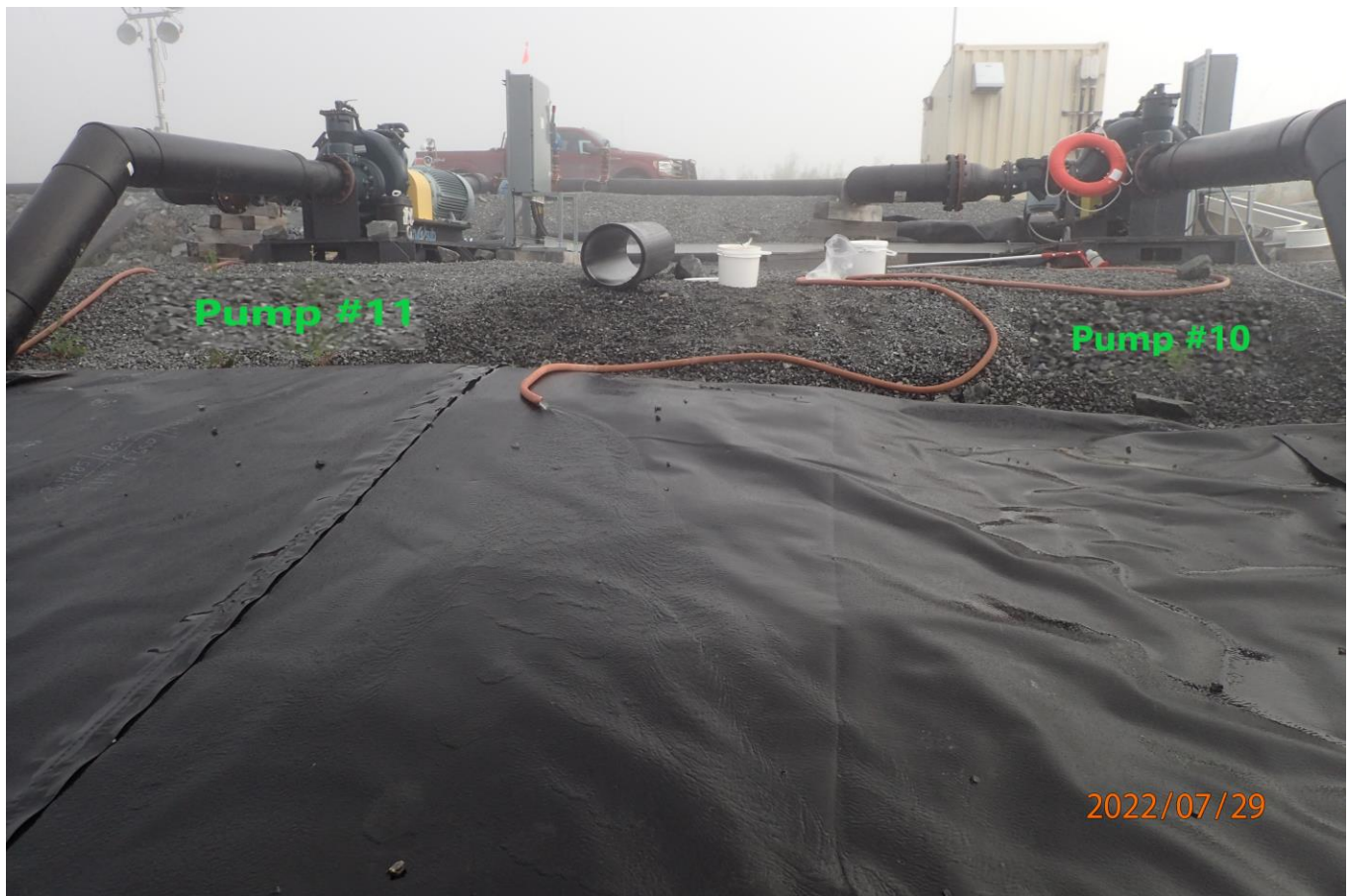
Photo 2: Outflow Basin Pumps
