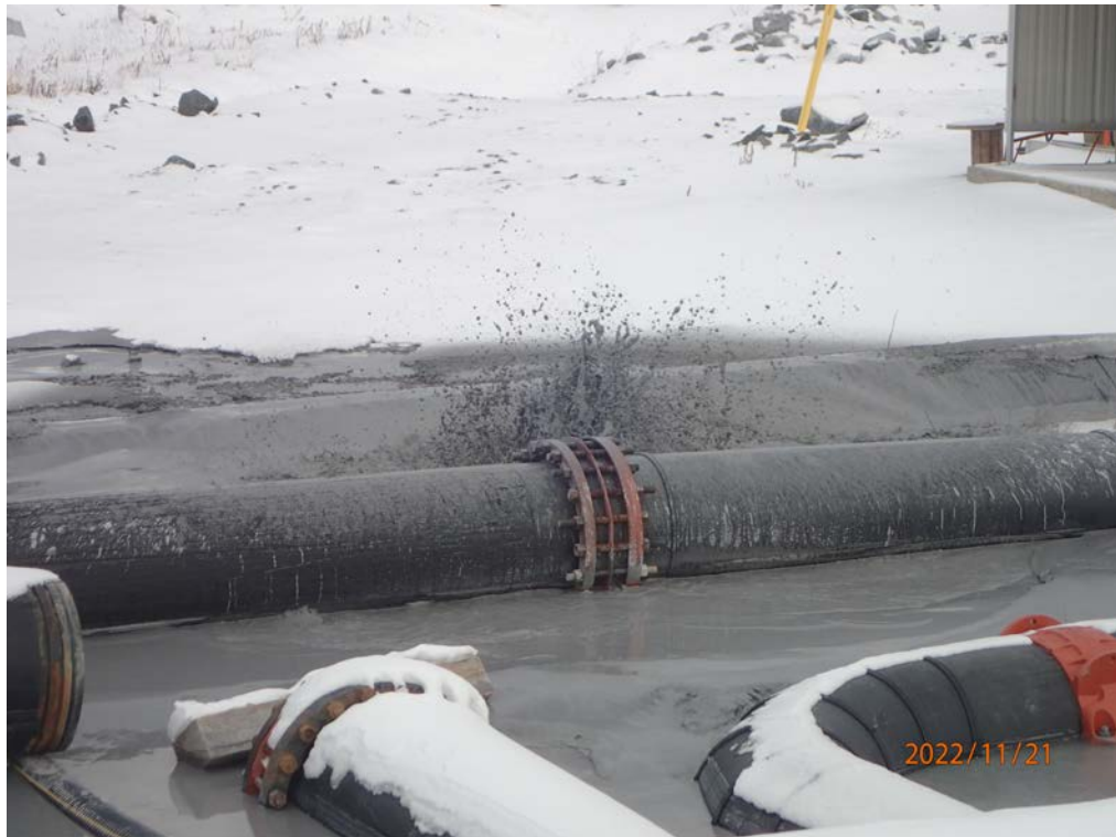
Photo 1: Leak at pipe connection
