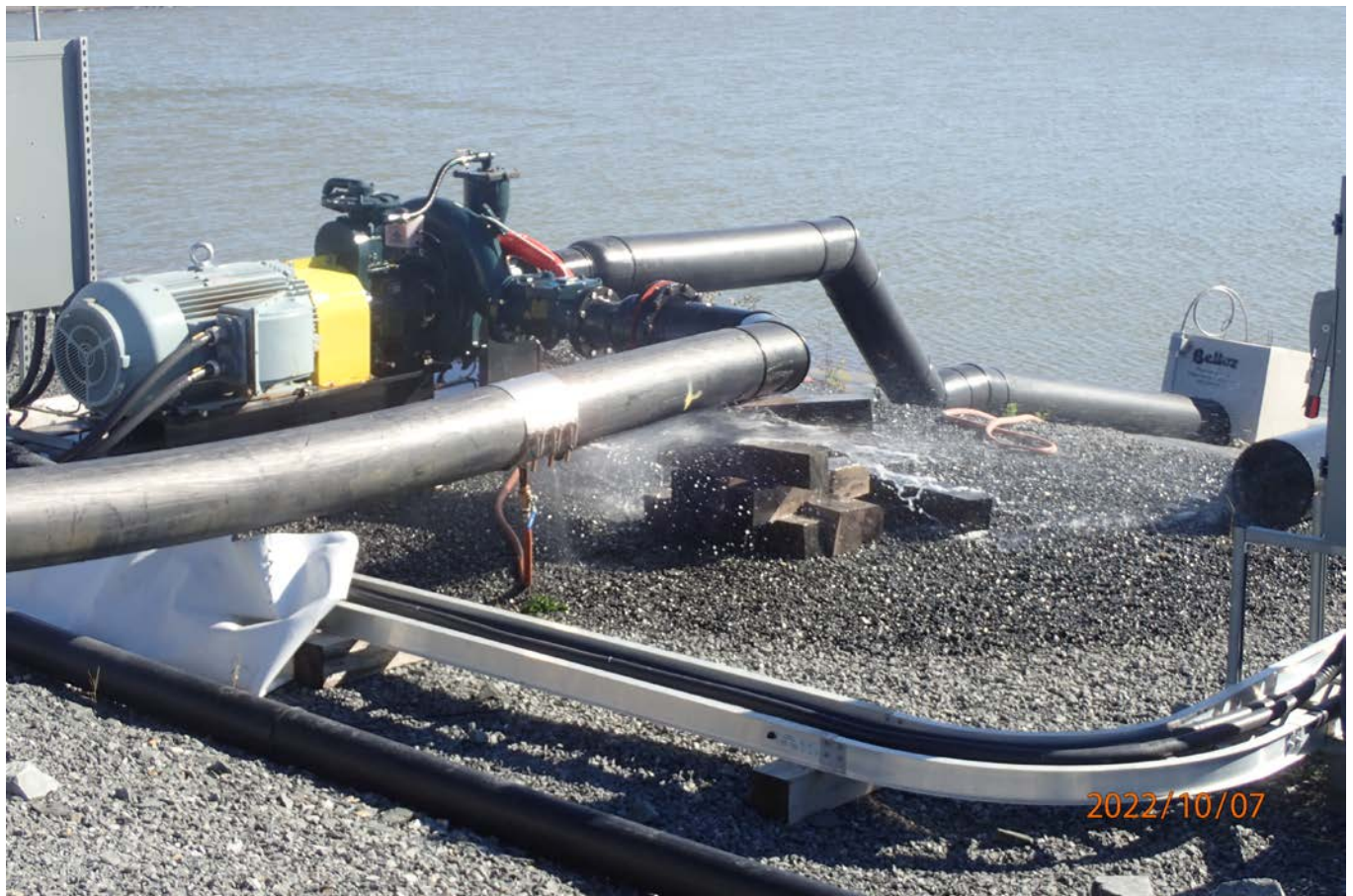
Photo 1: Leaking hugger clamp.
