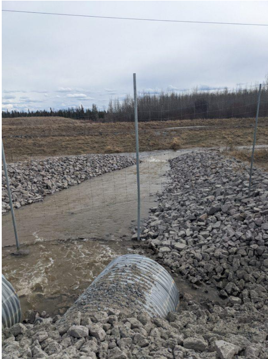
Figure 2 Turbid water observed travelling under Roan Road into West Creek Diversion.
