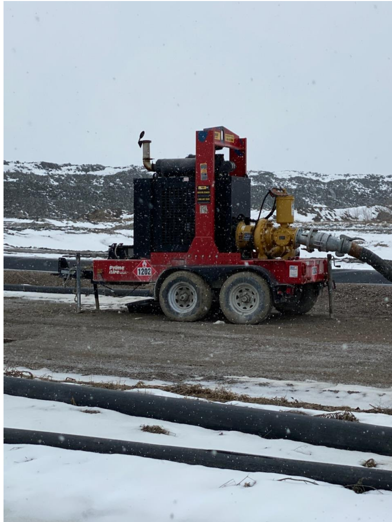
Figure 6 High-Volume pump installed to discharge water straight into tailings line and into the TMA.
