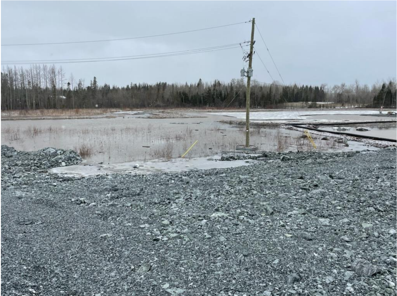
Figure 1 April 25, 2022 water build up around Seepage3.
